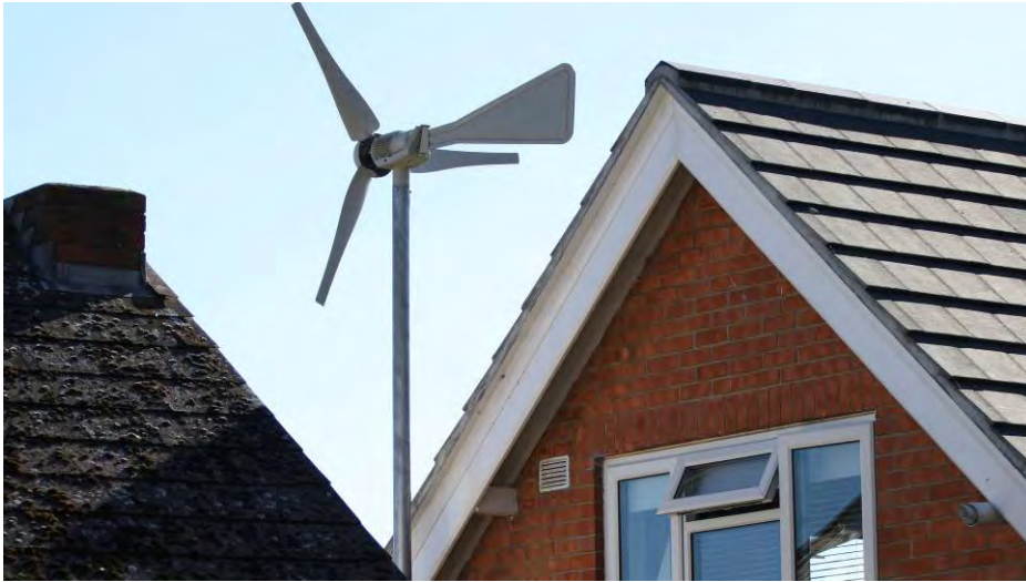
Alternative energy systems
