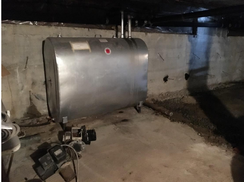
Photograph No.15: Heating oil AST on the ground floor of the apartment building
