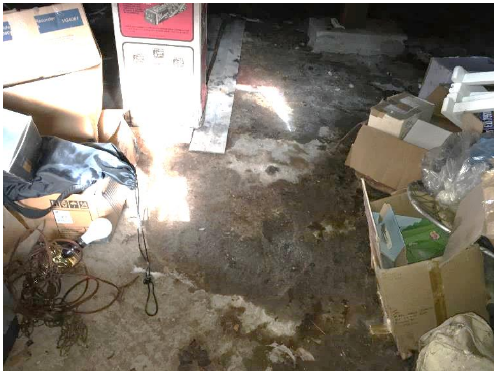
Photograph No.18: Staining on the floor of the crawl space under 1445 Burnside Rd W
