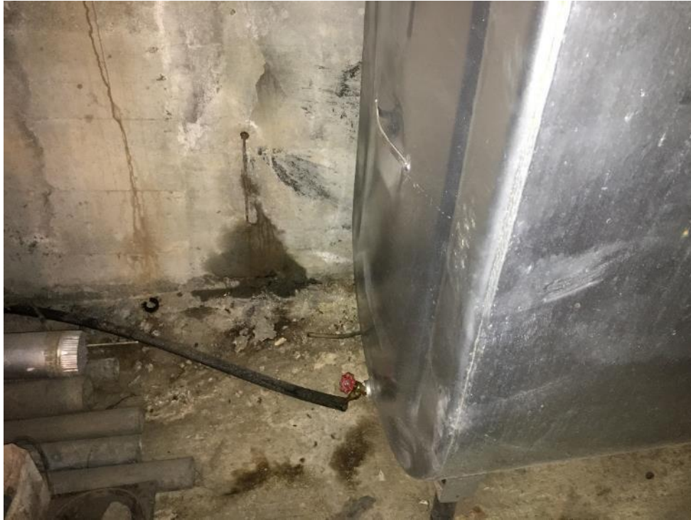
Photograph No.19: Staining under the valve of the AST at #3 Helmcken Rd
