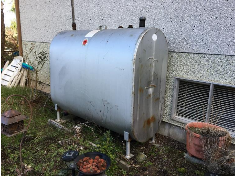
Photograph No.17: Heating oil AST on the west side of the house at 1449 Burnside Rd W
