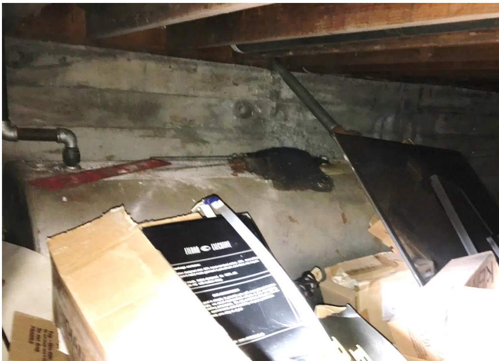
Photograph No.16: abandoned heating oil AST in the crawl space under the house at 1445 Burnside Rd W
