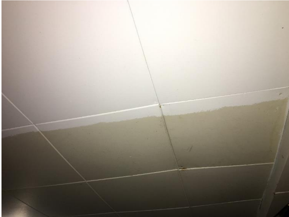
Photograph No.21: Example of ceiling tile that is suspect of containing asbestos
