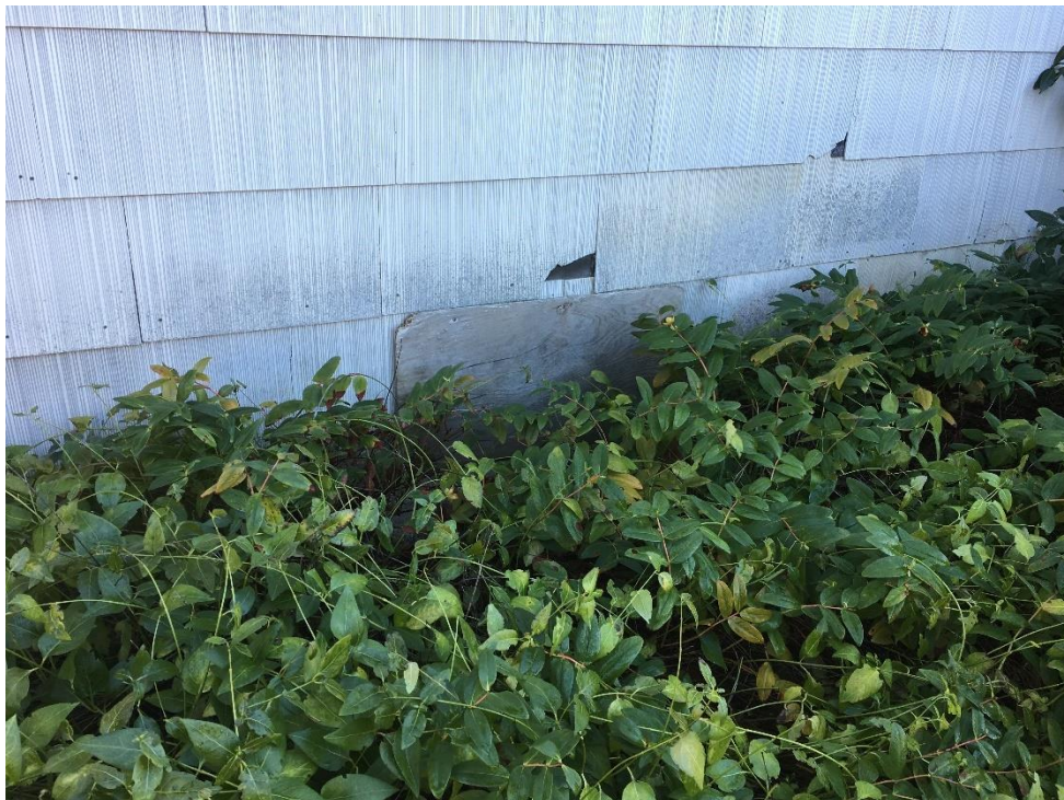
Photograph No.22: Asbestos cement siding on the house at 1447 Burnside Rd W
